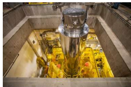
Tritium Extraction Facility Personnel Receive Irradiated TPBARs Shipped from Watts Bar in Preparation for Extracting Tritium for the Nation's Nuclear Deterrent
